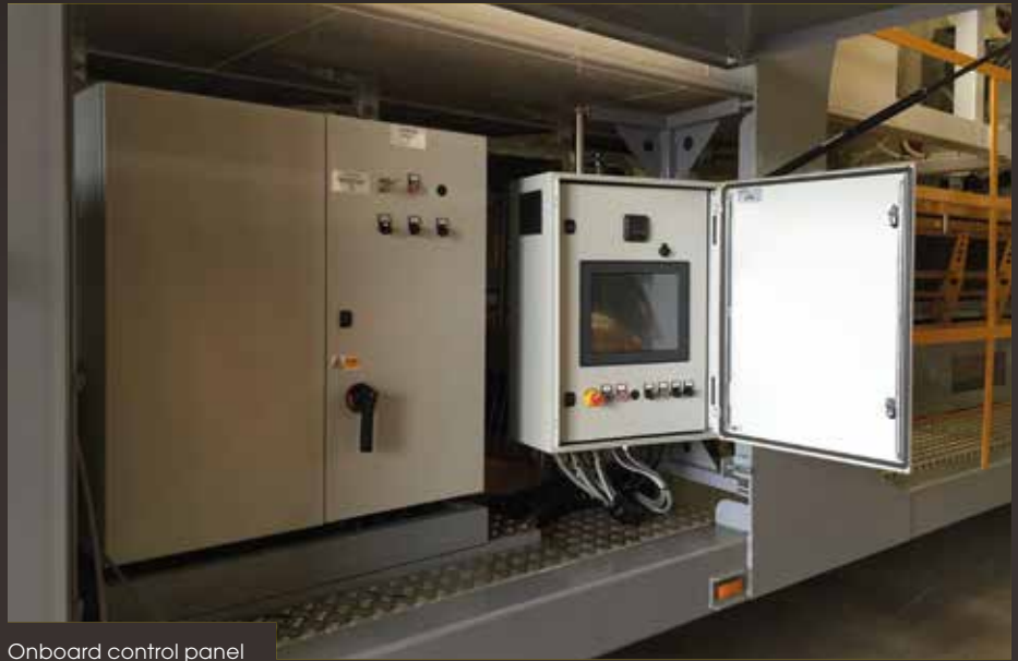
Onboard control panel
